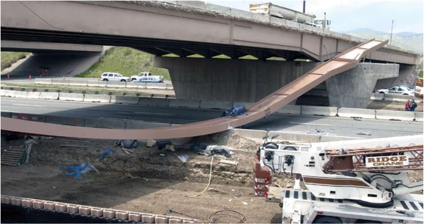
IN MAY 2004, THREE PEOPLE WERE KILLED WHEN A STEEL GIRDER FELL INTO THE EASTBOUND LANES OF I-70 IN GOLDEN, COLORADO.
